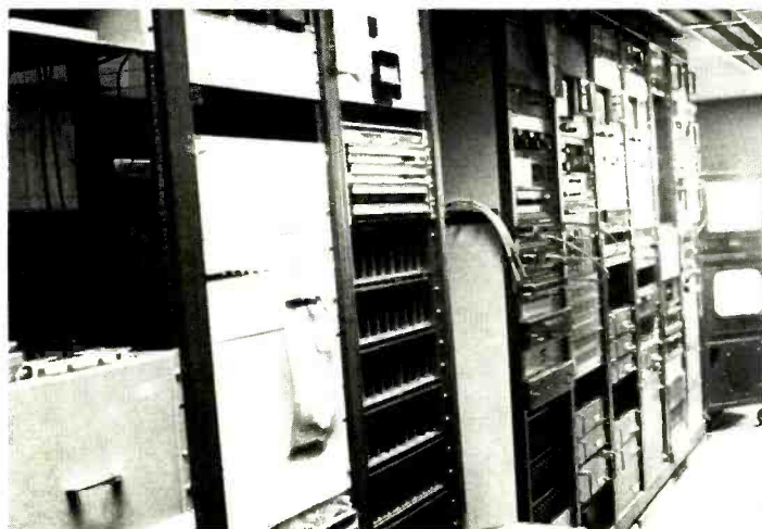
Tapes from portable equipment can be played on the Sony half-inch unit, left rack. There is a proc amp in second rack and a TBC to the far right.
