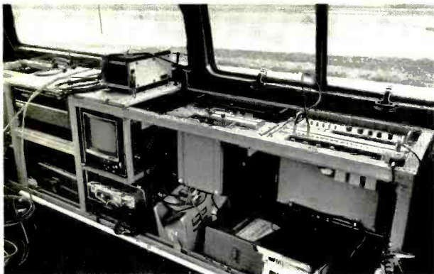
Inside the van is microwave video equipment, two-way radio communications gear, monitors, color bar test generator and time code generator. Some units have IVC BCR-100 recorders. Others work with Sony 3800s.
